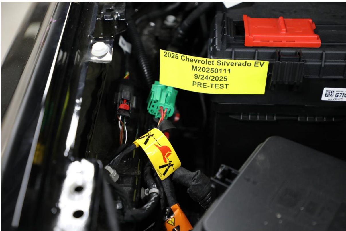
305-06 Manual High Voltage Service Disconnect in Place
